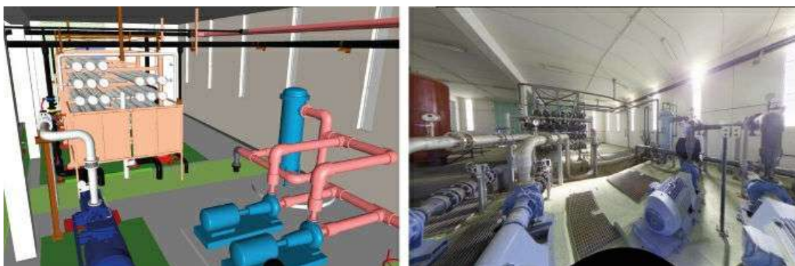
Advanced tertiary treatment for irrigation water at the Wastewater Treatment Plant (WWTP) of El Ejido, Almería.
